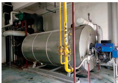
蚌埠食品廠節能器安裝 Installation of energy saver in Bengbu food factory
