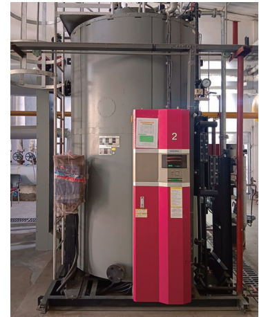
滄州肉品廠鍋爐遠程監管 Remote monitoring of boilers at Cangzhou meat factory
